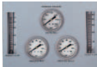
Pressure Gauges and flow meters
