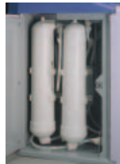
Inside of Diamond RO unit showing membranes
